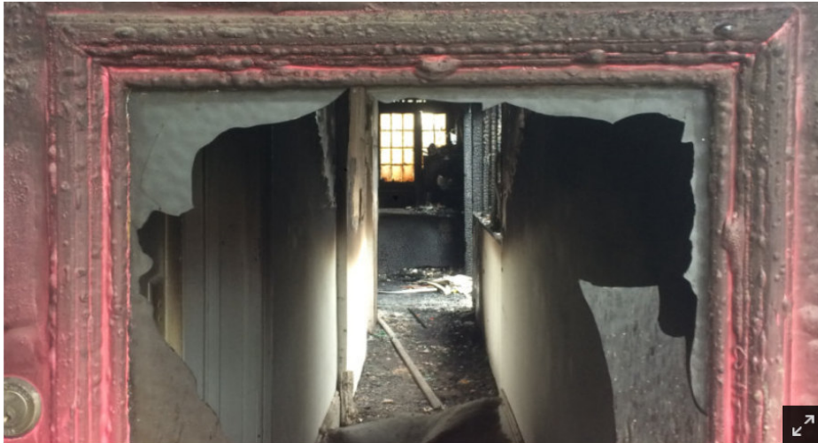
View of Melanie Sandford's home gutted by fire through the front door. MILO TAYLOR-WESTERMANN
