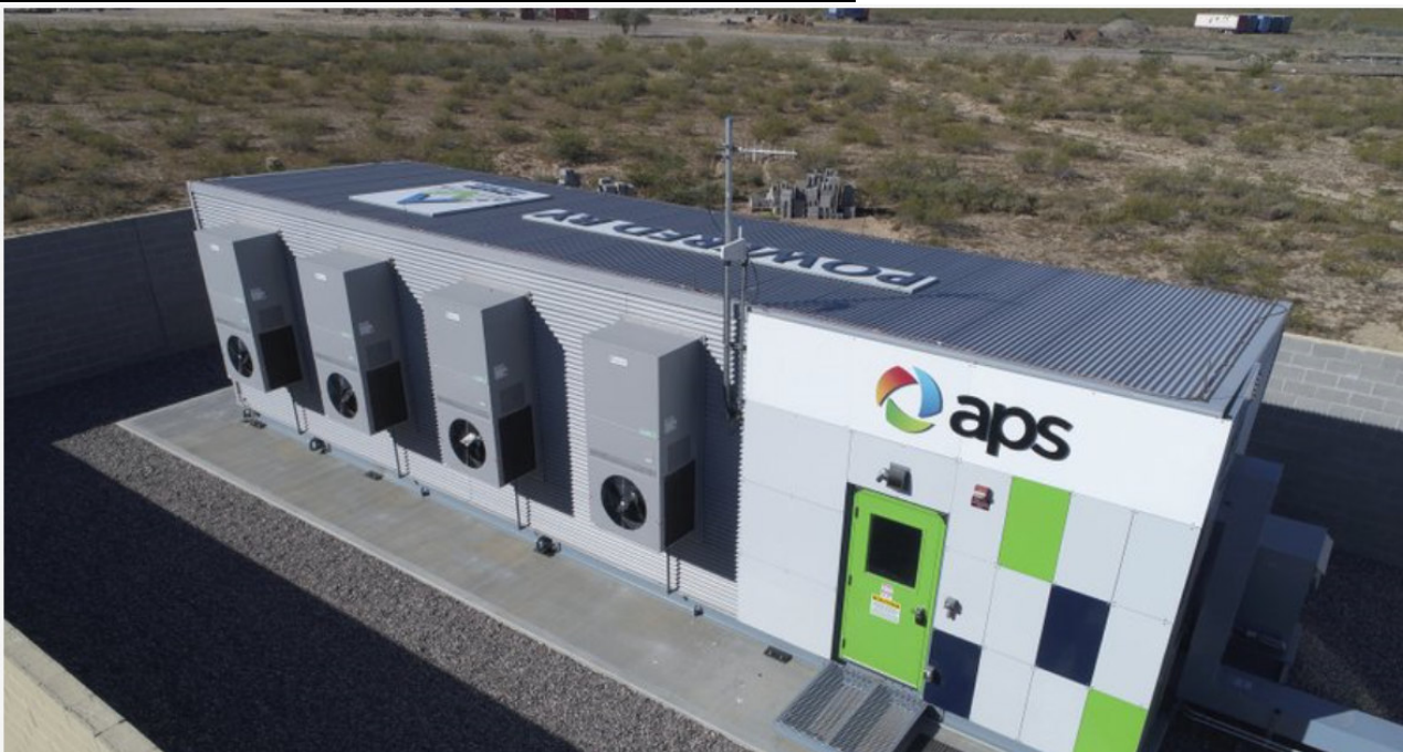
Figura 47. This photo taken in May 2017 and provided by Arizona Public Service shows the Festival Ranch 2 megawatt battery owned by Arizona Public Service near Buckeye, Ariz. An identical battery caught fire in
